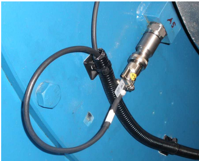
Sensor installed and wired at measuring location A5.
