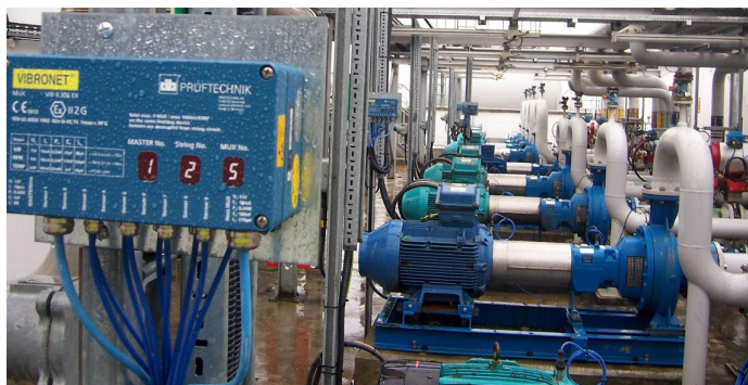
Typical MUX installations
