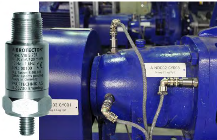
Monitoring vibrations with VIBROTECTOR
